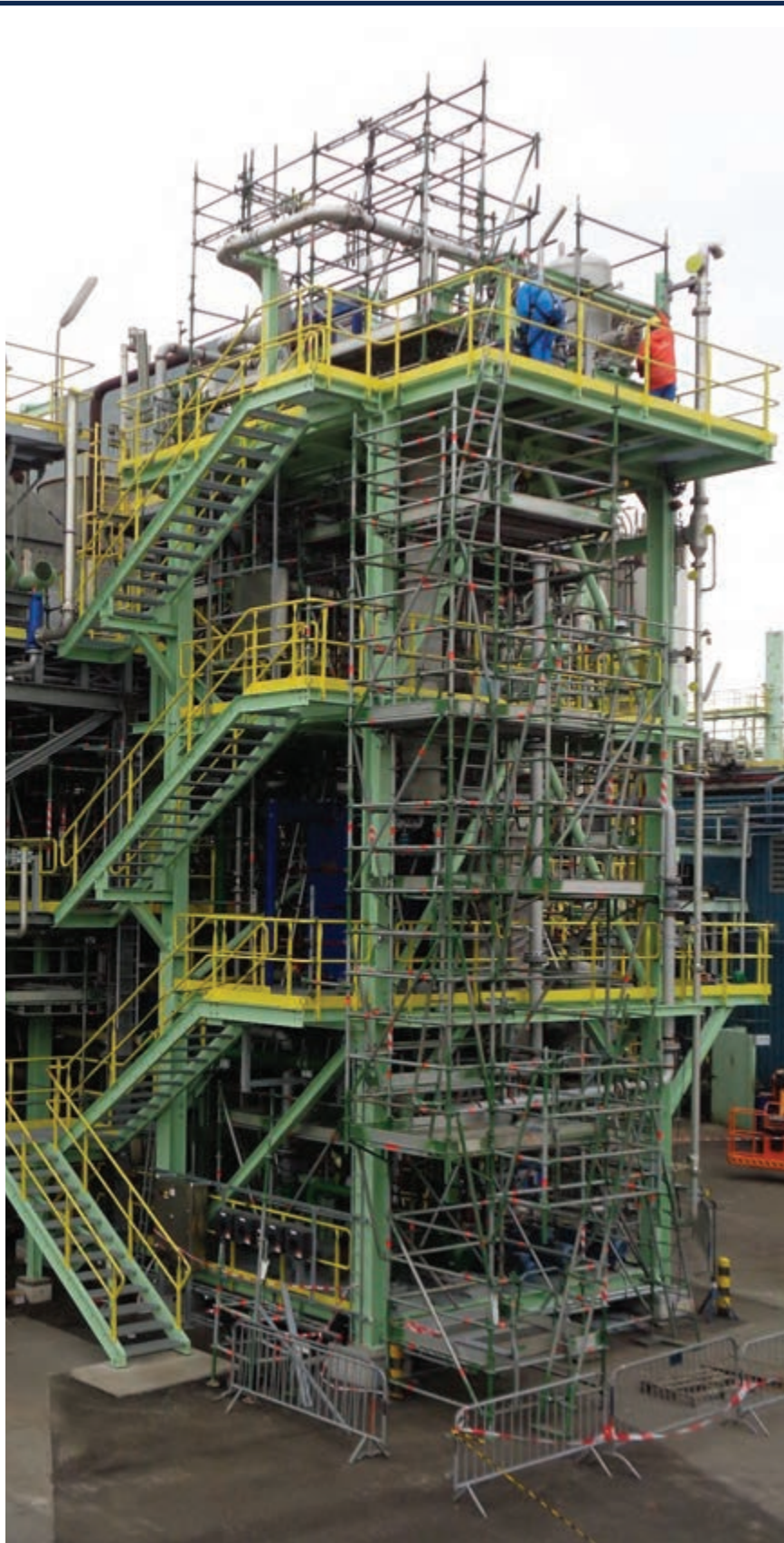
Qpinch's pumps are being added to a Borealis LDPE unit in Antwerp
